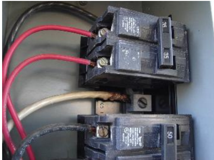
Over heater electrical conductor
